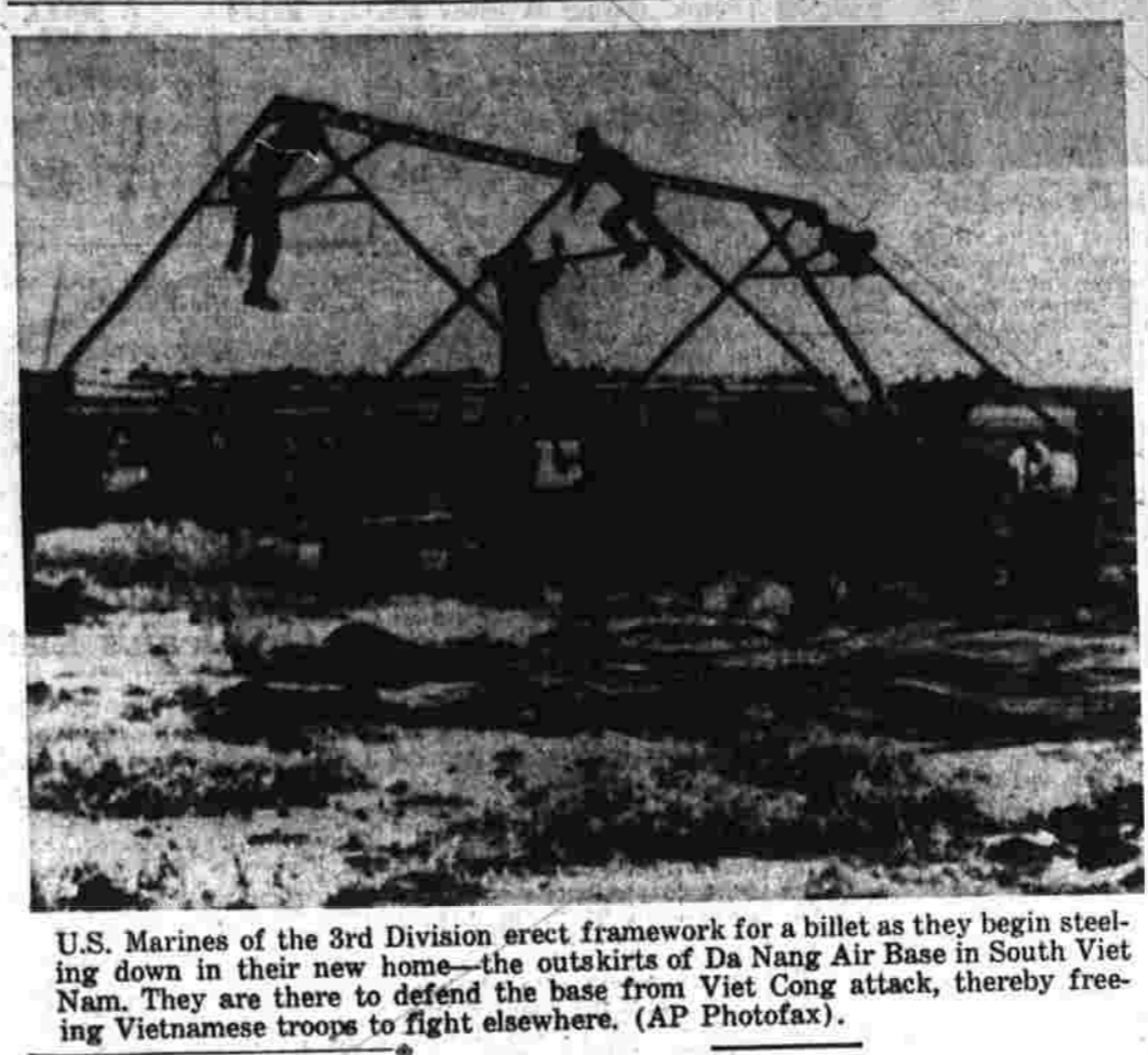
U.S. Marines of the 3rd Division erect framework for a billet as they begin steeling down in their new home—the outskirts of Da Nang Air Base in South Viet Nam. They are there to defend the base from Viet Cong attack, thereby freeing Vietnamese troops to fight elsewhere. (AP Photofax).
