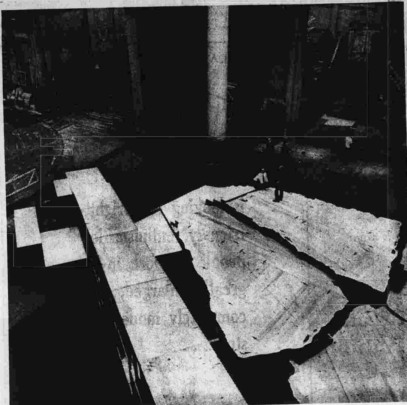
Part of the T-shaped stage complex where platforms are being built for "Elektra."
