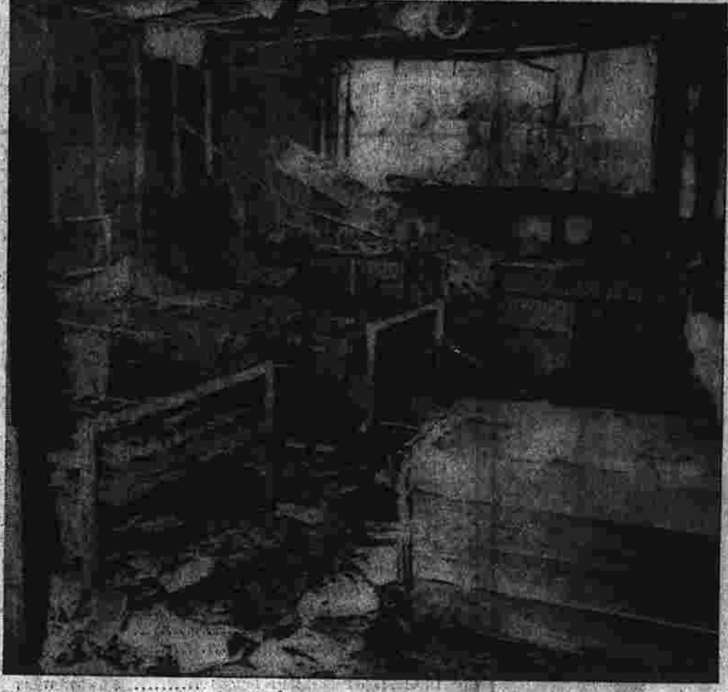
This charred basement room indicates the intensity of a fire that killed nine persons in a Cornell University residence hall early this morning. Eleven others were injured in the blaze. (AP Photofax)
