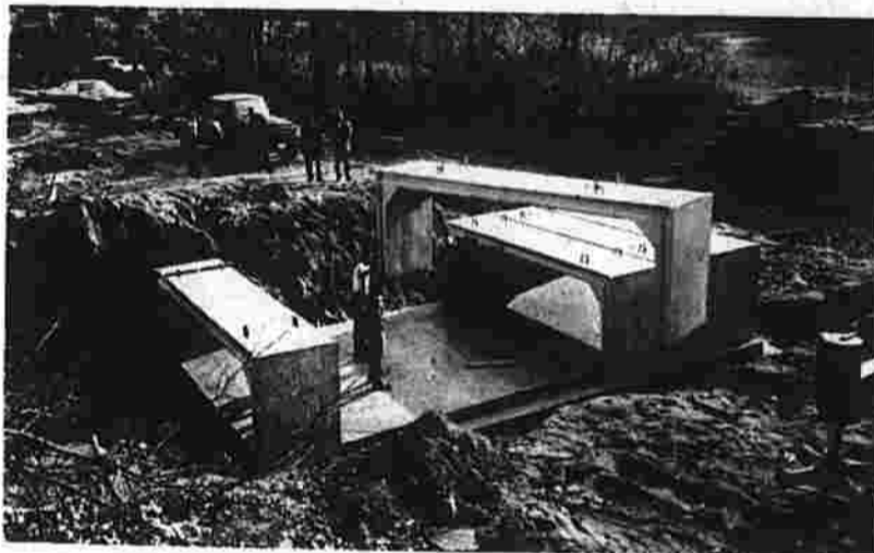
The Bidwell St. bridge over Folly Brook had to be rebuilt in November 1975 after being washed out in a torrential rainstorm earlier in the fall. One of eight sections of pre-cast concrete culvert is shown here after it was installed.
