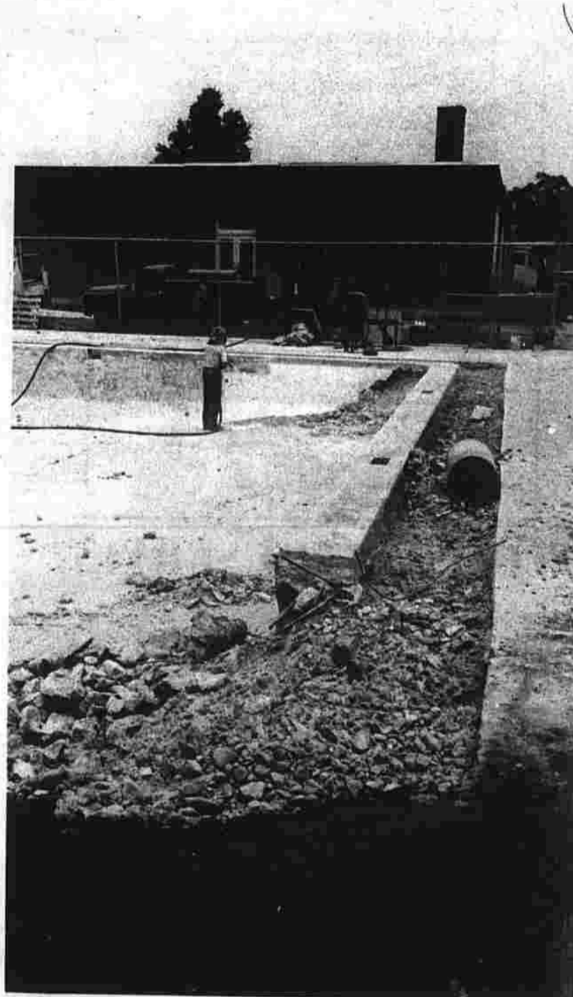
The Verplanck pool underwent extensive renovation. Piping for the circulation system had deteriorated. In the renovation process a ramp was provided for handicapped persons. The pool opened late but was used a great deal.
