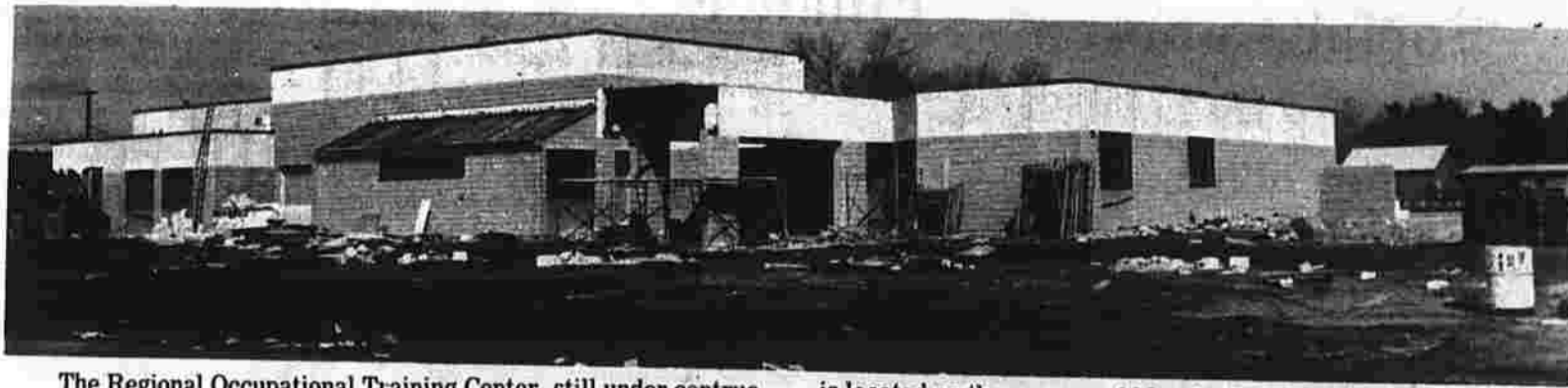
The Regional Occupational Training Center, still under construction when this picture was taken, opened this fall. The $1.4 million regional facility for special education vocational training
