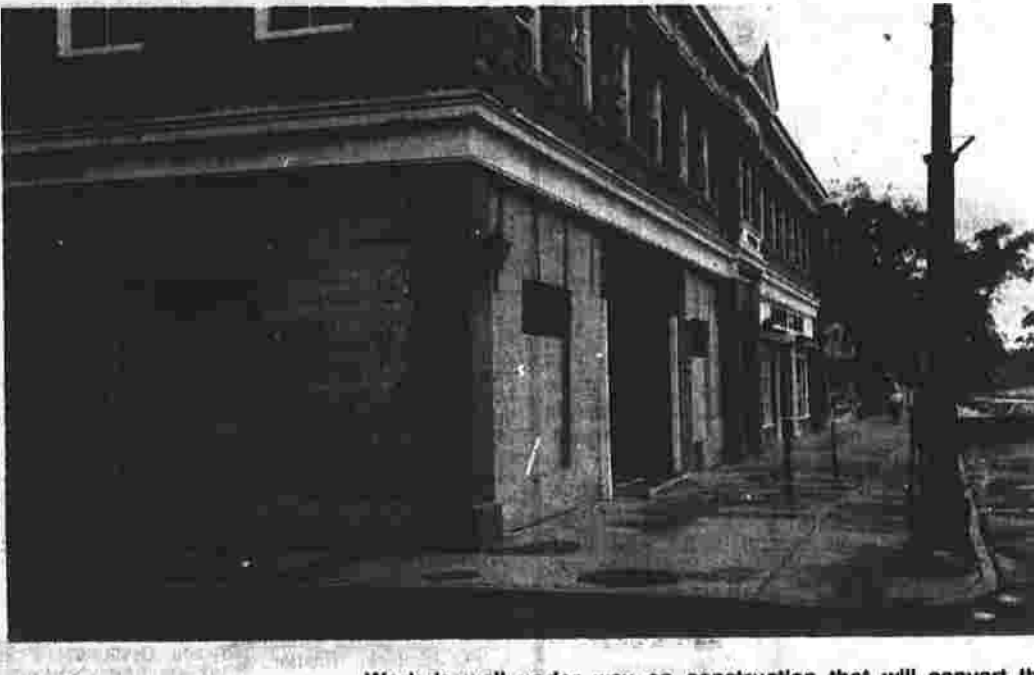
Work is well under way on construction that will convert the former House and Hale department store on Main Street to business condominiums, which will be called One Heritage Place. Plans call for display windows being boarded up, as the exterior masonry of the three-story, historic building is restored.
