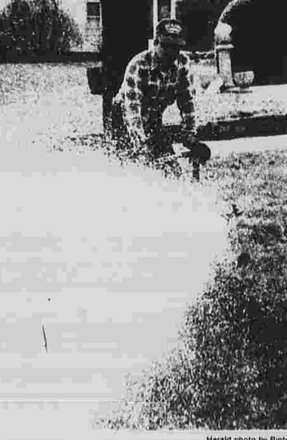
Flushing, required each year by state regulation, removes sediment from the lines.
